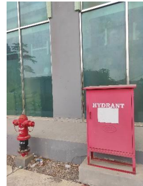
Gambar 1.15 Sistem Proteksi Kebakaran Hydrant
